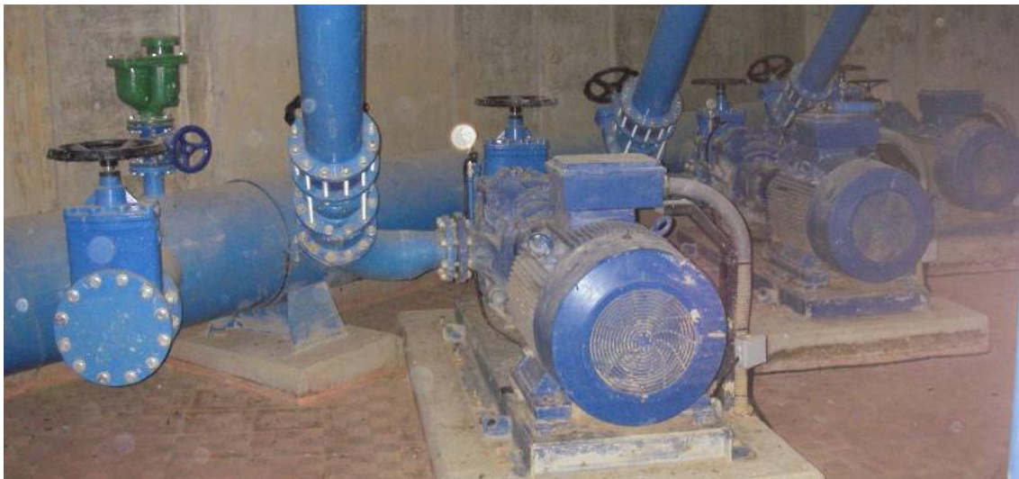
Ilustración 7. Existing pumps with intake for reversible pump.
