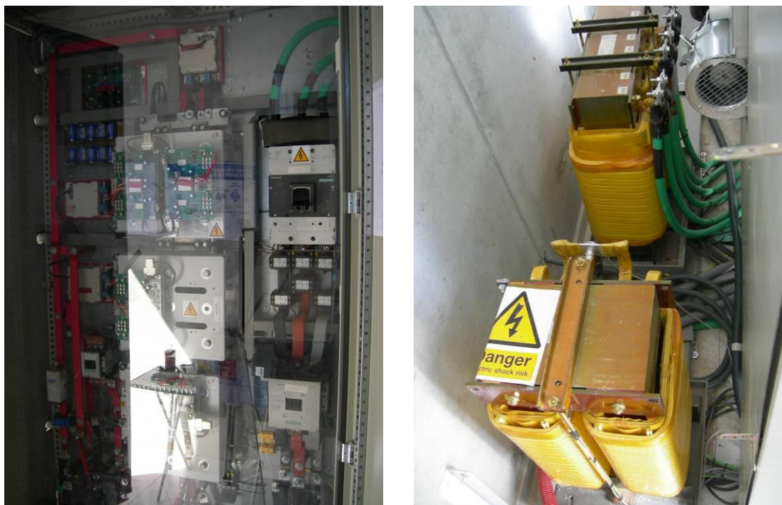
Ilustración 8. Power cabinet (left) and grid-side filters (right).
