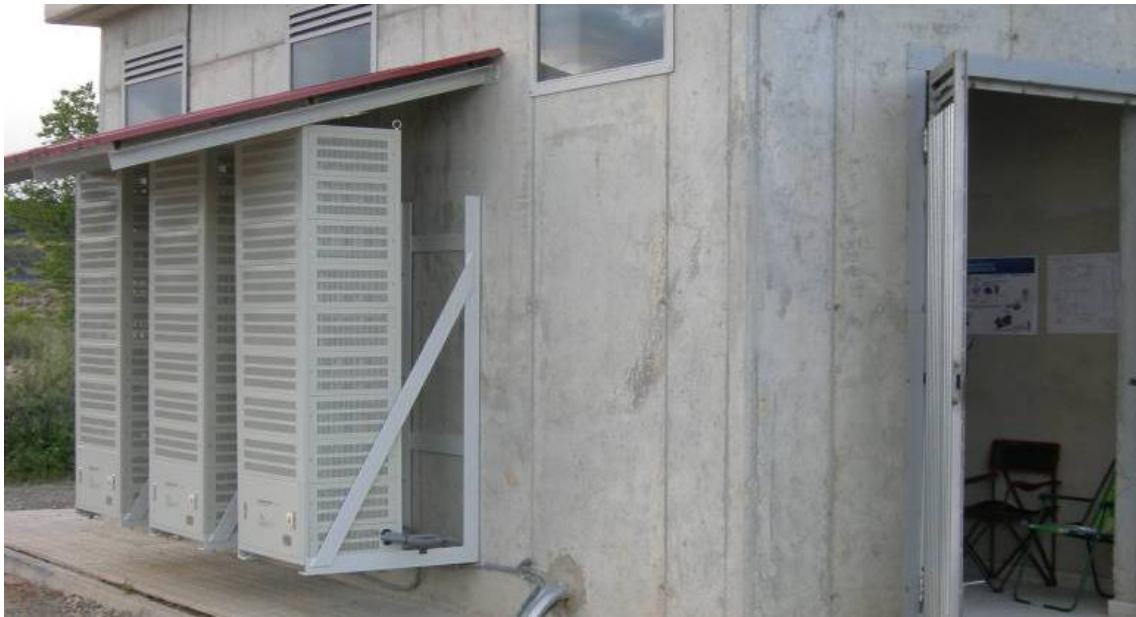
Ilustración 10. Chopper resistor cabinets, situated outside the building.
