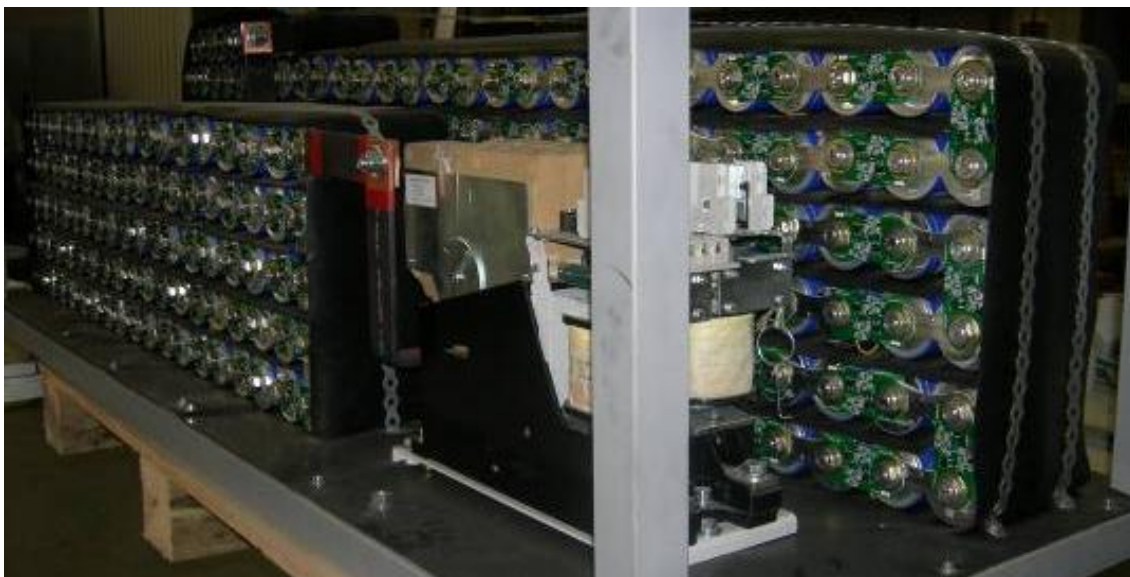
Ilustración 11. Detail of the cabinet with ultracapacitors.
